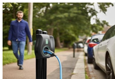
On street AC Charging
